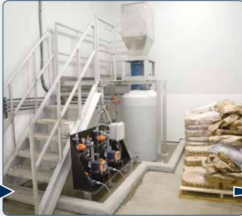
A coagulant called ISOPAC and soda ash, used to raise the pH, are added to the raw water to facilitate treatment.
