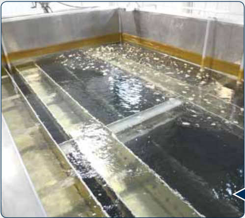
The water is then pumped into a dual media filter tank, trickling through anthracite coal and sand layering its bottom.
