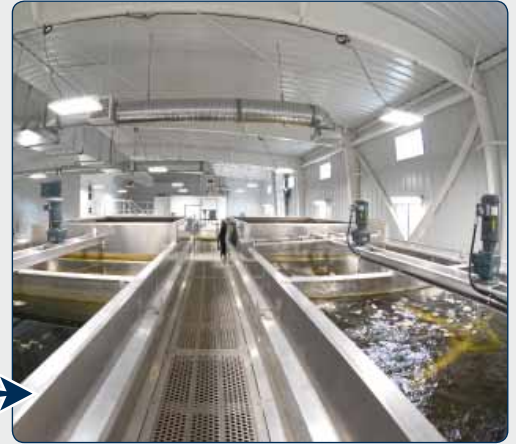
Mixing helps to ensure the chemicals are evenly distributed through the water. Note how only one 'train' (right) is active.
