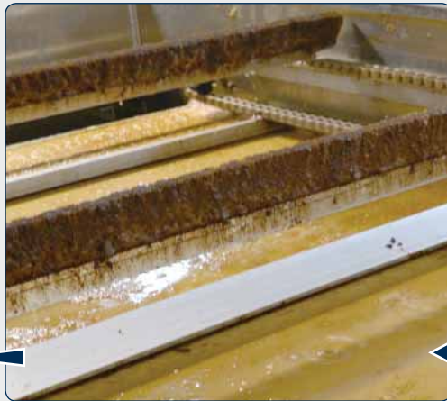
Brushes scoop the scum from the surface of the tank while the treated water is collected in a perforated pipe at the bottom.
