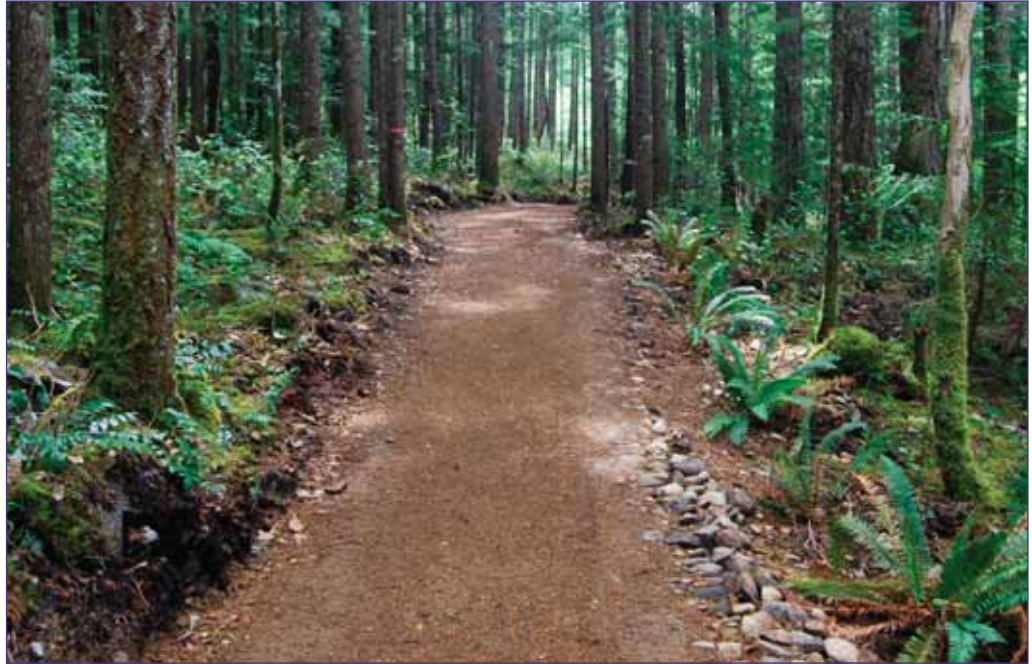
Vandals removed boulders guarding an entry point to this section of the recently constructed Suncoaster Trail. RCMP believe the boulders were removed by ATVers looking to gain access.
