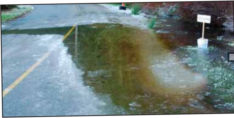
JANUARY: Someone used humour to voice their frustration over this chronically flooded section of Hotel Lake Rd.
