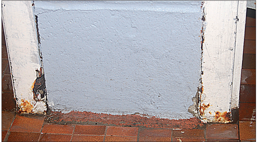
After years of painting and patchwork repairs, the aquatic centre is overdue for some TLC.
