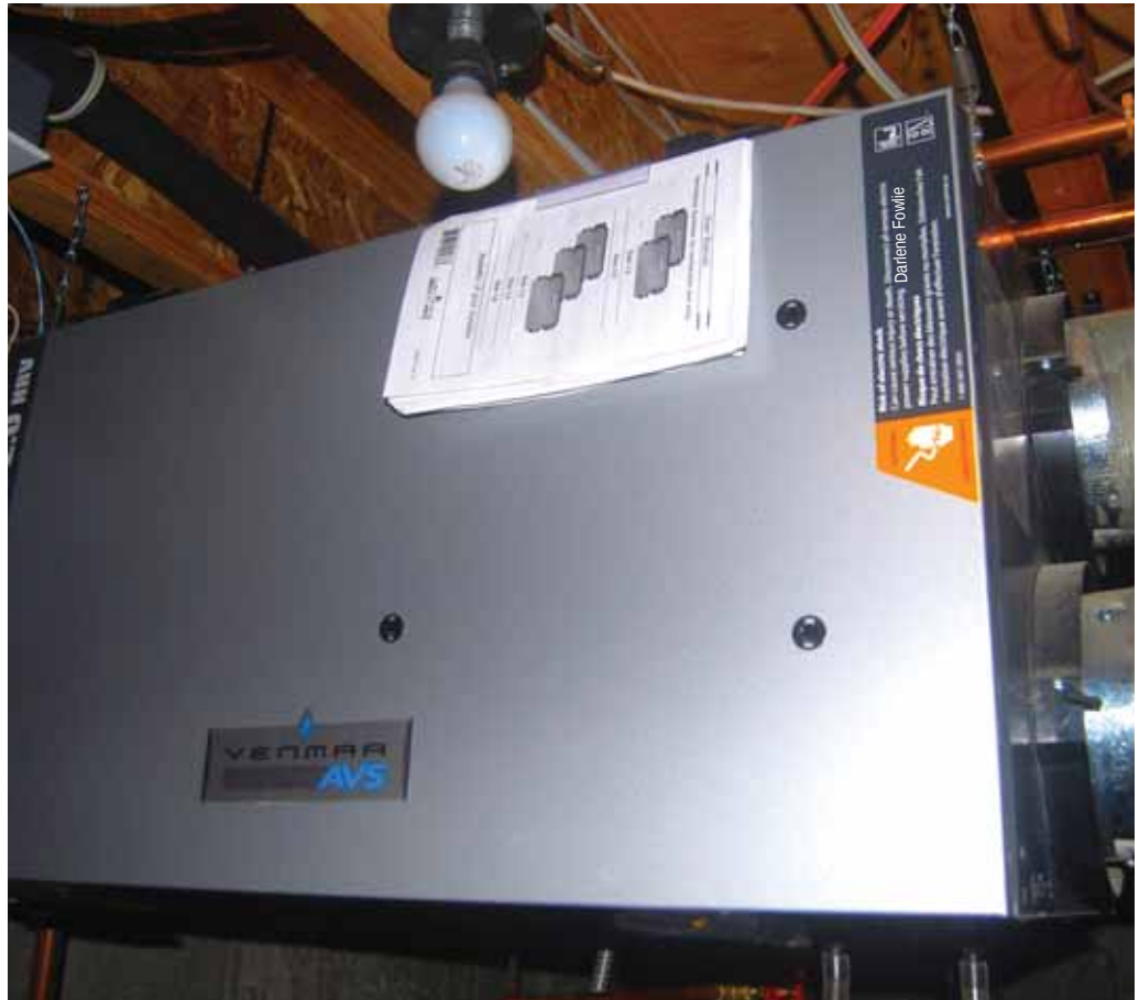
Mechanical air filtration systems like this one are becoming increasingly common in modern, airtight homes.
